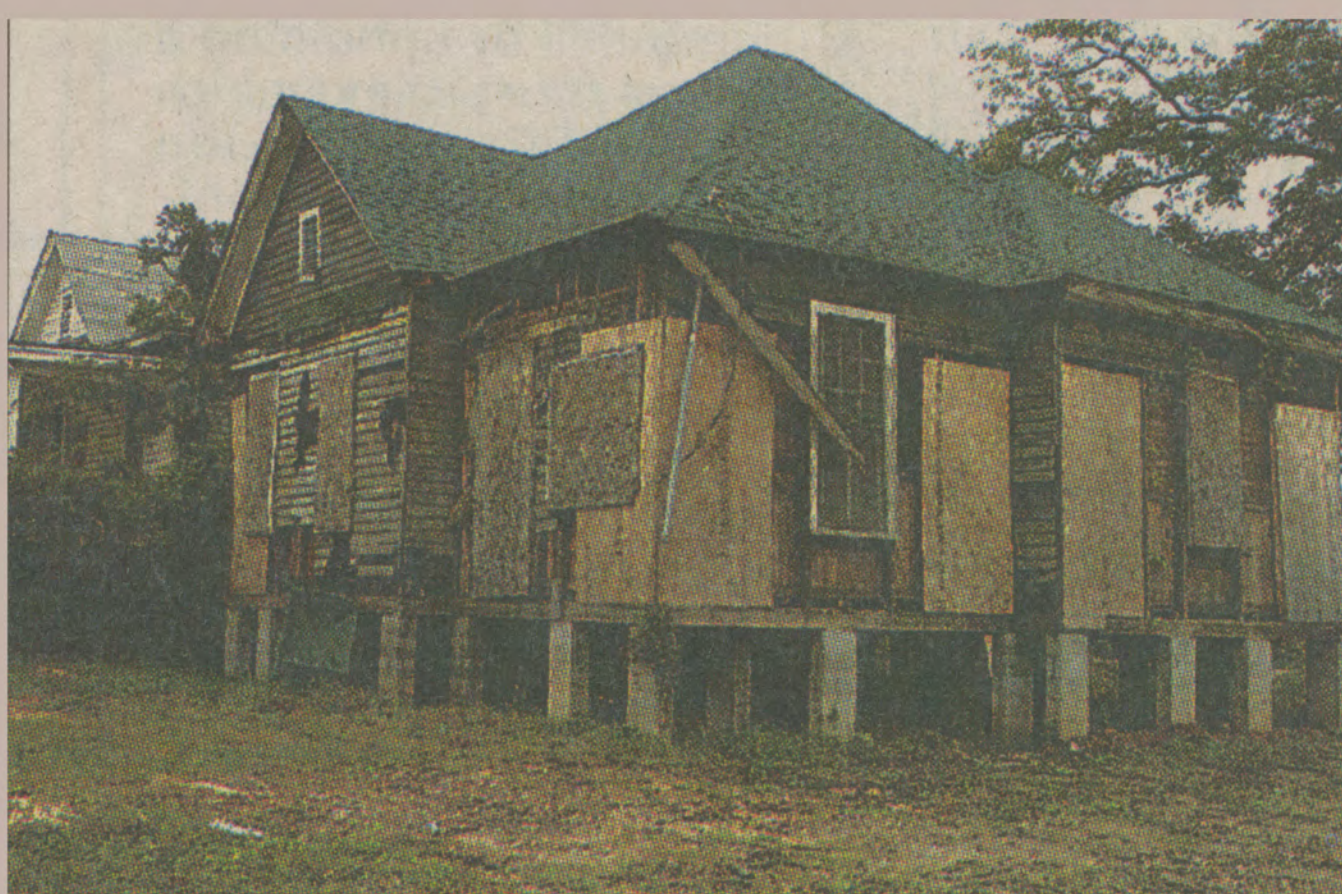
Nat King Cole House, 2008 Asbestos siding removed before the house was relocated.
